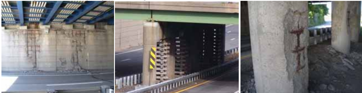
Pier and wall deterioration examples
