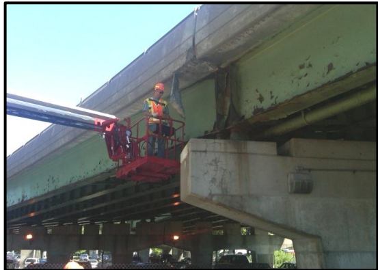
I-81 Bridge Condition - Failure
