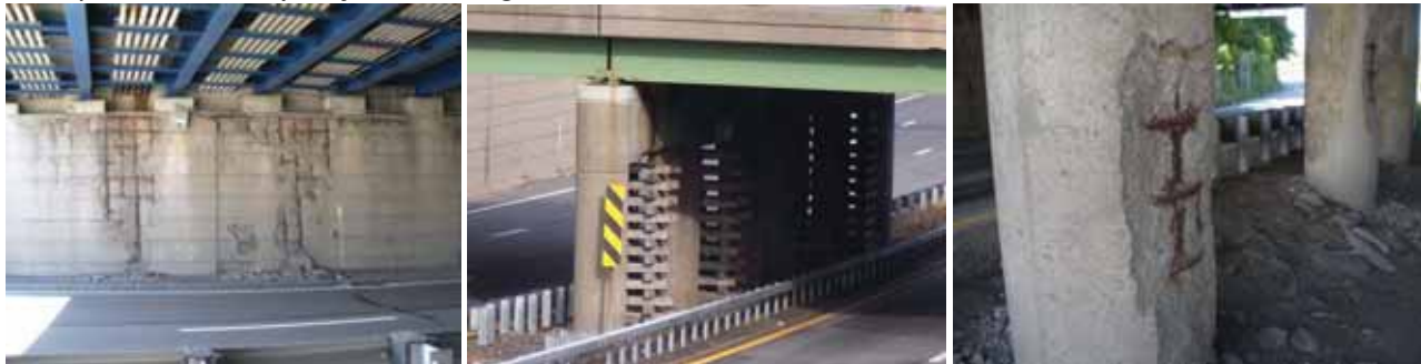
Pier and wall deterioration examples
