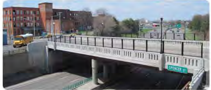
The Spencer Street bridge is an example of a project subject to the Categorical Exclusion process.
