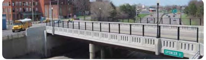
The Spencer Street bridge is an example of a project subject to the Categorical Exclusion process.
